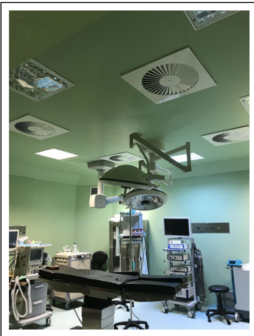
Figure 2. The operating room with conventional airflow systems (CAS-OR).
